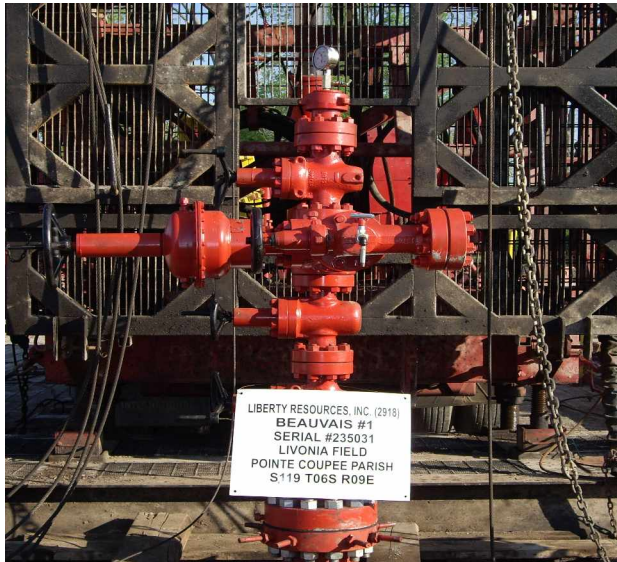
WELL HEAD – BEAUVAIS #1
